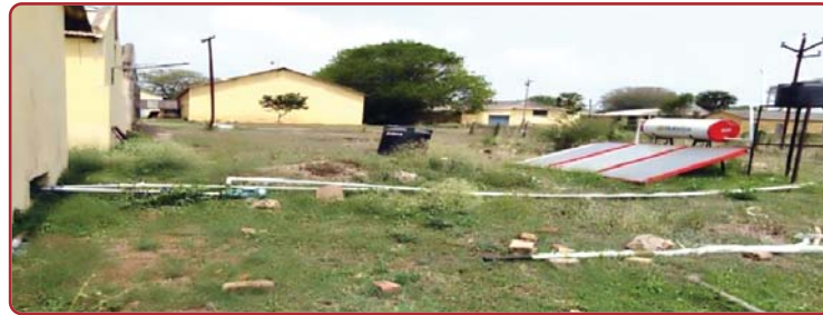
Solar Hot water circulation system
